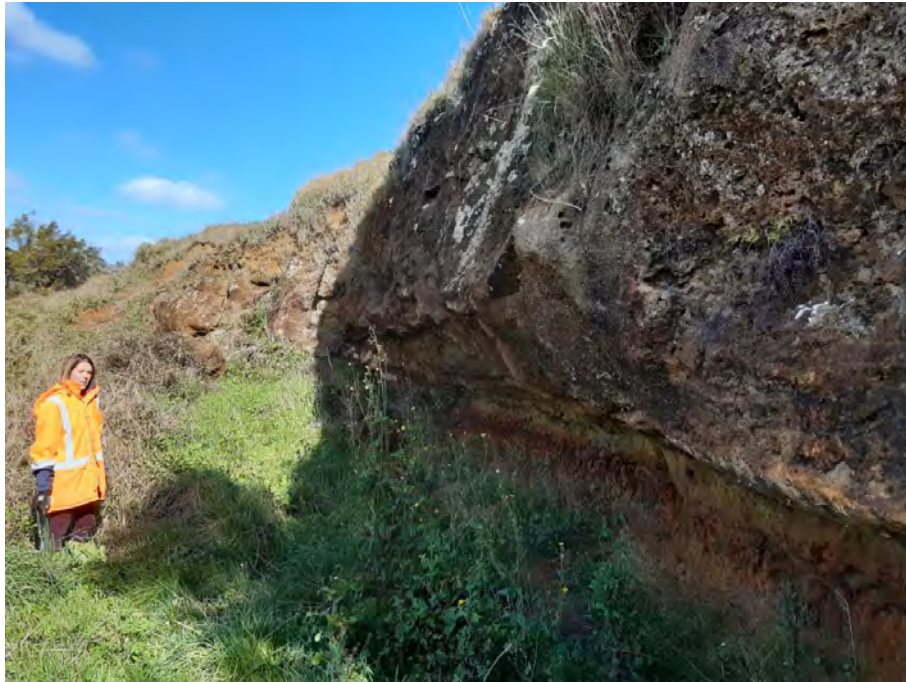
Photo 3: Weakly cemented sand horizon underlain by interlayered silts and sands. The weakly cemented sand is relatively resistant to erosion whereas the weaker interlayered beds beneath have been preferentially weathered. Although the strength of the weakly cemented sand horizon does vary across the site, this stratification is believed to underlie much of the ridge the proposed works are to be undertaken.
